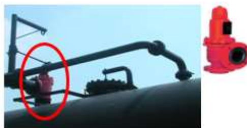
Gambar 10. Safety Relief Valve.
