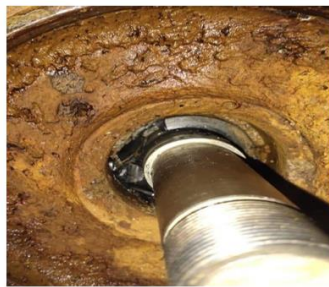
Gambar 3. Kerusakan Mechanical seal .
