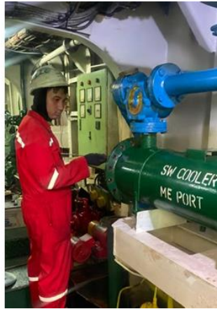
Gambar 5. Fresh Water Cooler
