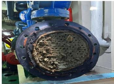
Gambar 2. Fresh Water Cooler
