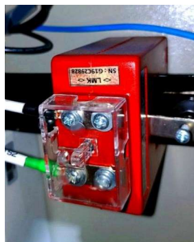
Gambar 6. Current Transformers (Transformator Arus)
