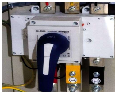
Gambar 2 Saklar Utama (Load Breaker Switch)
