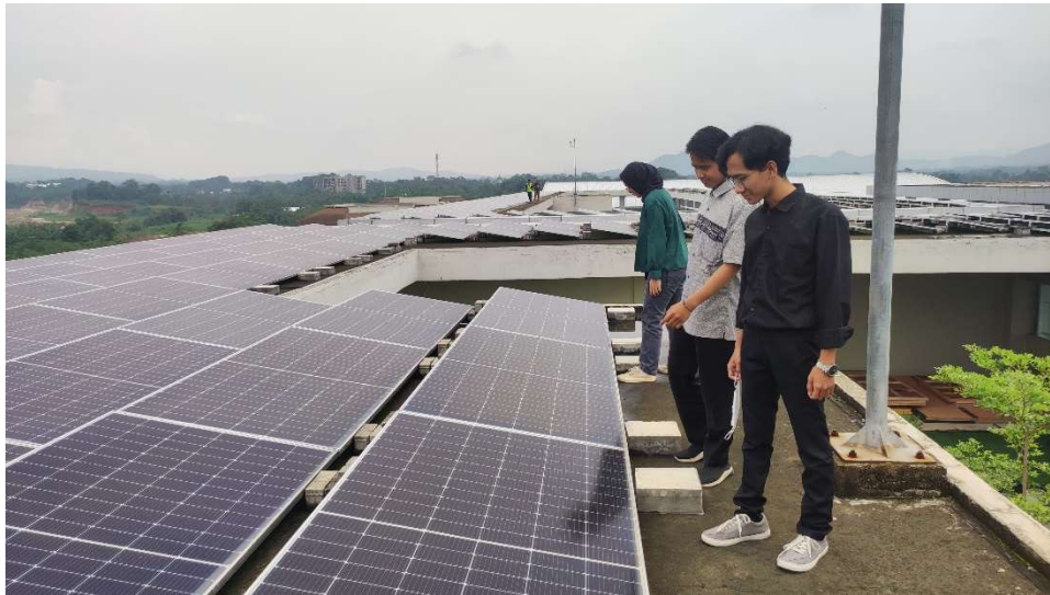
Gambar 2. Panel surya untirta
