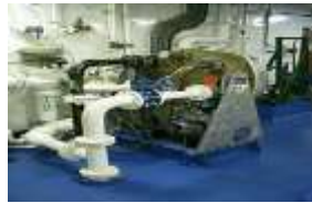
Gambar 1 Fresh Water Generator
