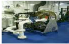
32 Gambar 1 Fresh Water Generator
